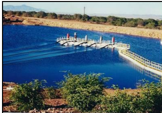
Fiberglass walkways, and pump barges
