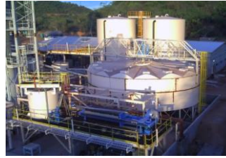
Tank & clarifier covers
