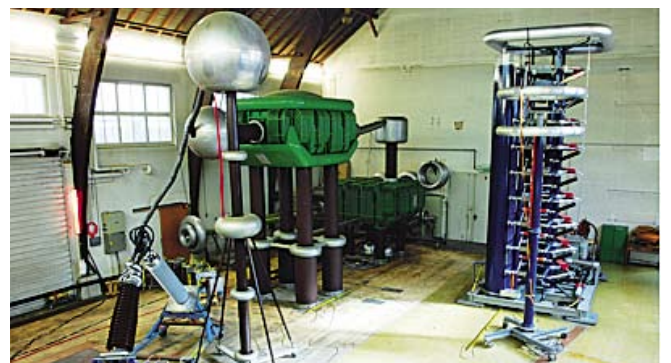
High voltage laboratory at Brugg Cables
