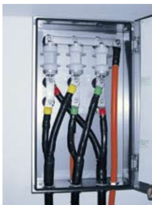
Disconnecting link box
