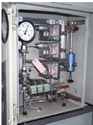
Pressure control cabinet of an oil-filled cable system
