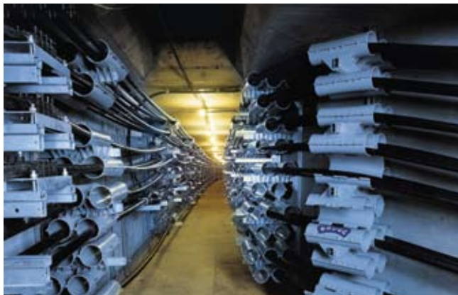
Proper mounting of cables with cable clamps of the Briport system in a concrete tunnel
