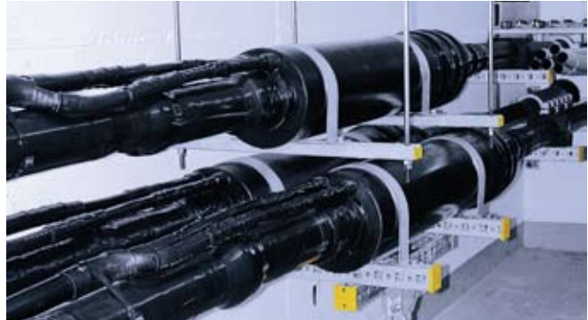
Joints with Cu-tube and HDPE coating in a concrete tunnel
