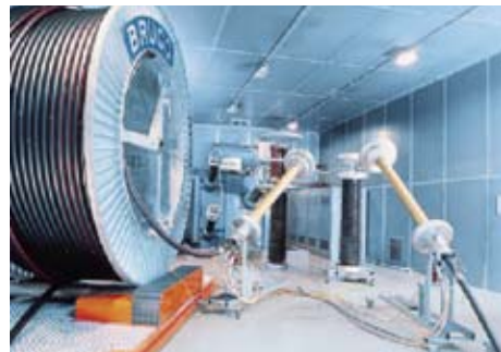
Brugg Cables' modern, fully screened test room for AC voltages up to 600 kV
