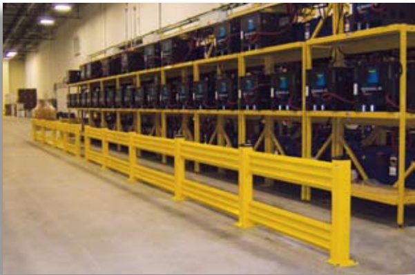
Guarding battery racks
