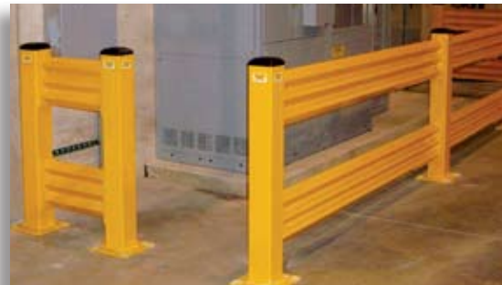
Guarding electrical panels
