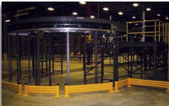
Guarding overhead conveyor
