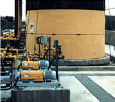
Centrifugal pumps transfer sodium hypochlorite from storage to day tanks for an odor control system.
