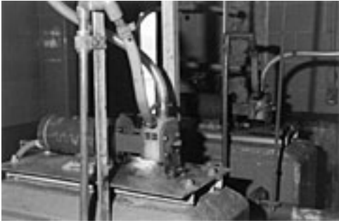
Flexible liner pumps, driven by variable speed motor, automatically feed sodium hypochlorite into wastewater.
