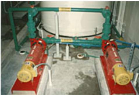
Polypropylene centrifugal pumps feed sodium hexametaphosphate from storage tanks to an injector in an influent pipe.
