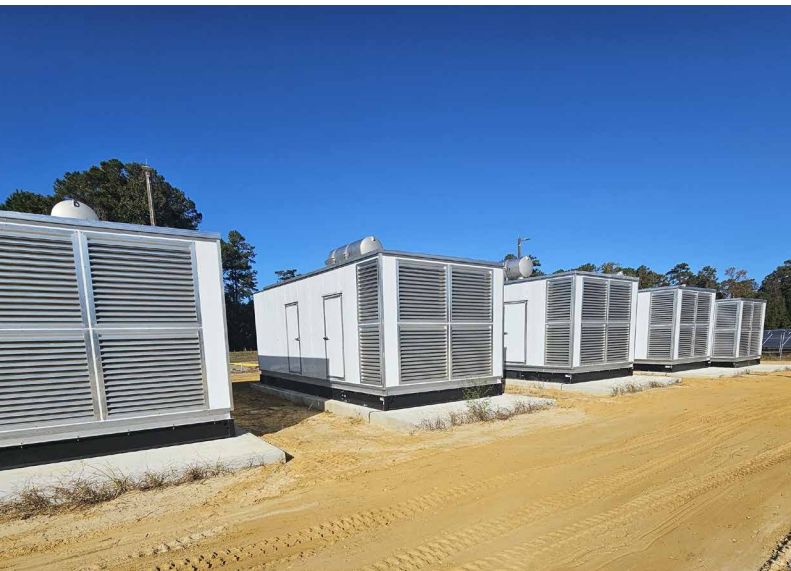
Powering through, no matter what! This microgrid will provide power to support the full load of Camp Johnson, located on Marine Corps Base Camp Lejeune, even if access to the main grid goes down. (Photo Credit: Craig Frank, Sain Engineering Associates)
