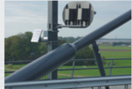
Installed External Damper
