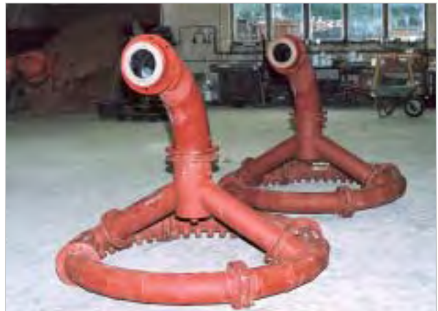
Pneumatic piping components used in a separator at a cement plant.
