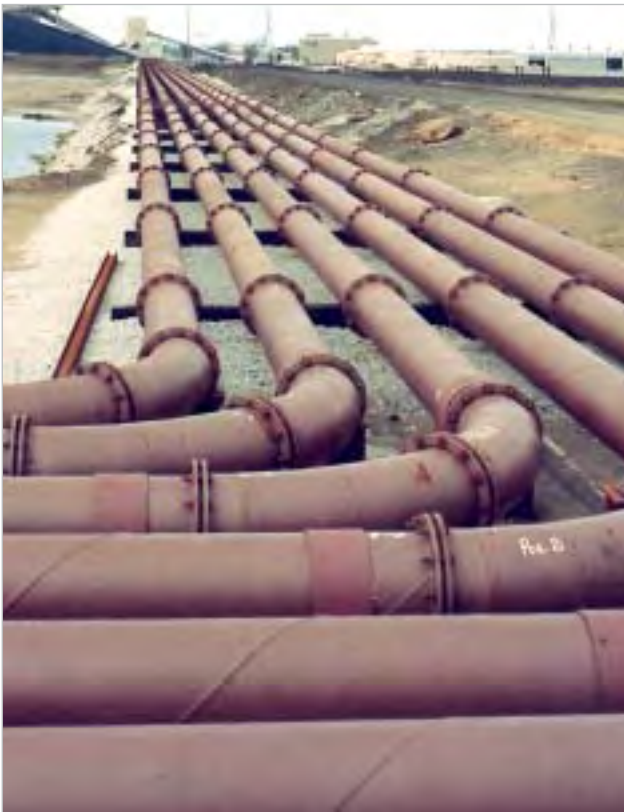
With lifetimes of more than 30 years, ABRESIST pipelines have been used for the hydraulic conveying of ash on all continents. This plant in the U.S. has over 10,000 meters of 294 mm ID pipe in service.
