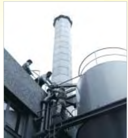
Costs go up when the repair location is difficult to reach.
