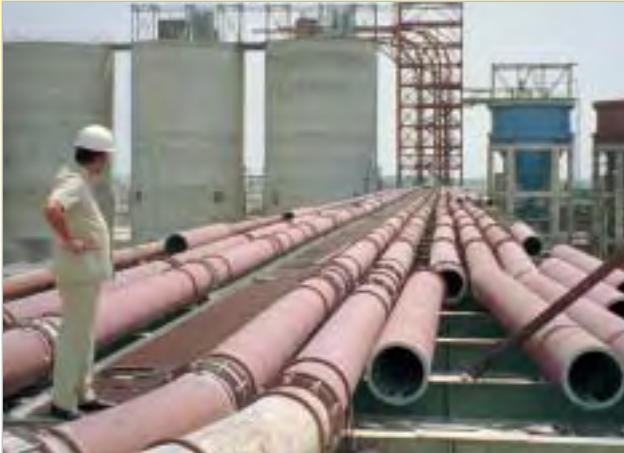
Hydraulic ash conveying at an Indian coal fired power station (four units 250 MW each).
