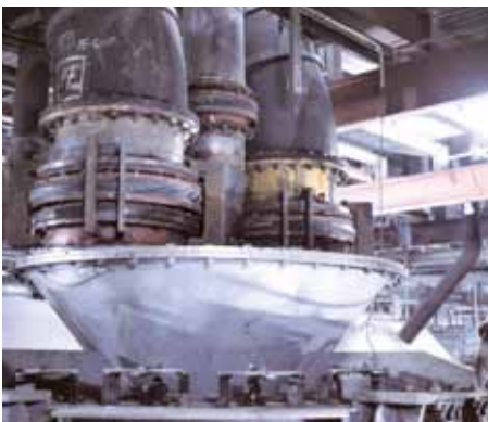
Discharge pipes - position 1.
