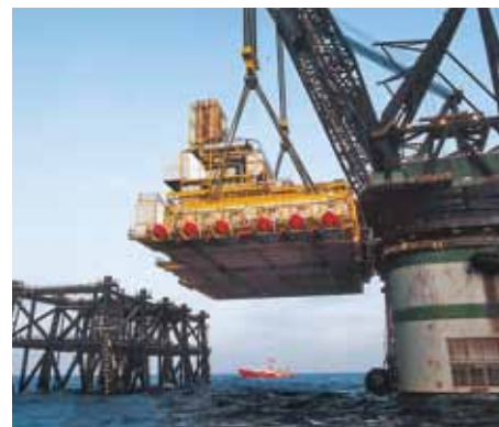
The piper feed unit equipped with Fluastal® Fabric Joints on the gas turbine exhaust.
