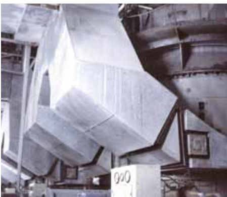
Primary air intake - position 2.
