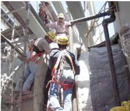
KE® Fabric Expansion Joint installed over the manifold.
