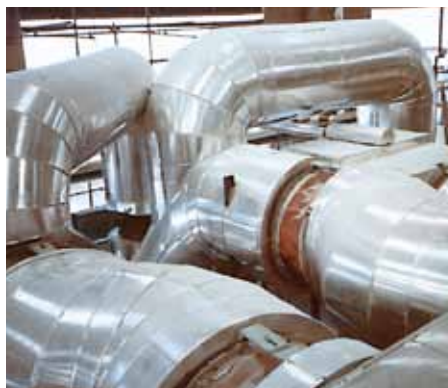
Installation of KE® Fabric Expansion Joint in a pulp and paper mill.
