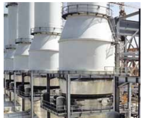
Gas Turbine System.
